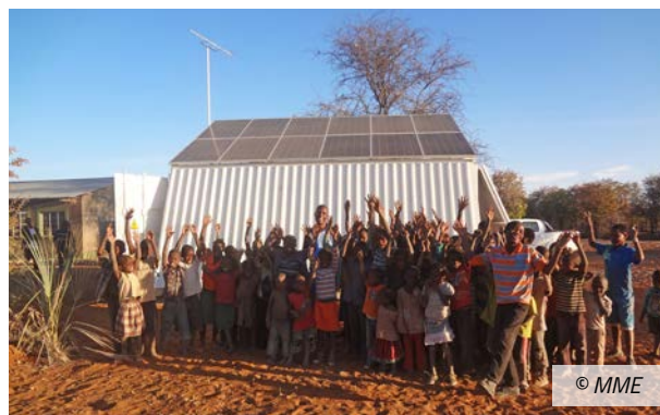
Containerized PV System improving access to energy for government institutions and households in Namibian rural areas.
